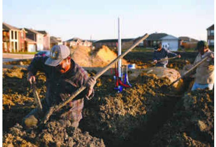
Silvano Perez (left) preps the foundation for a house at Windmill Farms, near Forney
